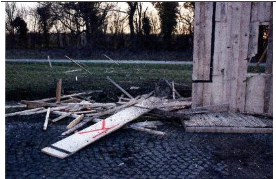
Figure 28 — The screen and sidewalk at the location of the NIK shop after the explosion
