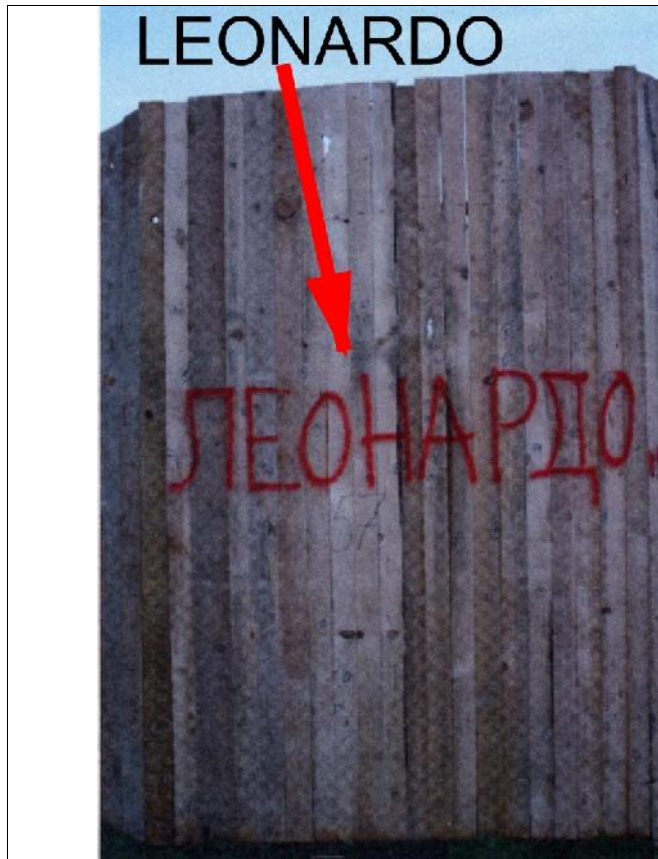
Figure 37 — Screen (of corner part of the building) housing the Kapija STR and cafe Leonardo after the experimental explosion
