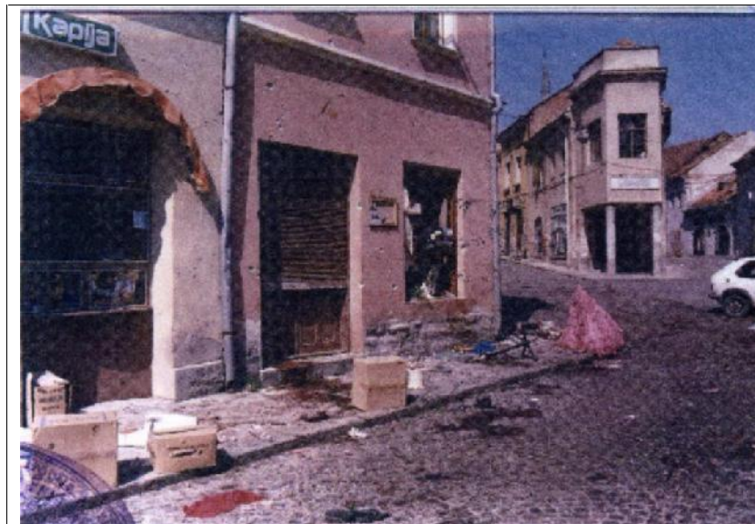
Figure 35 — Building of the Kapija STR after the explosion on 25 May 1995
