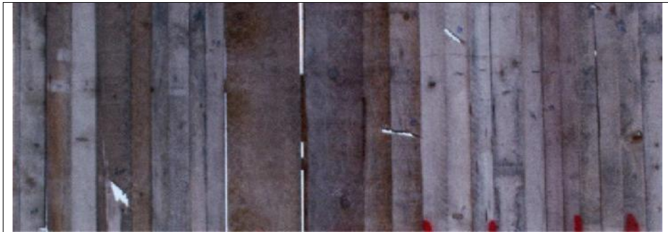
Figure 34 — Detail of the screen (wall) of the building of the Kapija STR with visible elongated perforations made by projectile fragments
