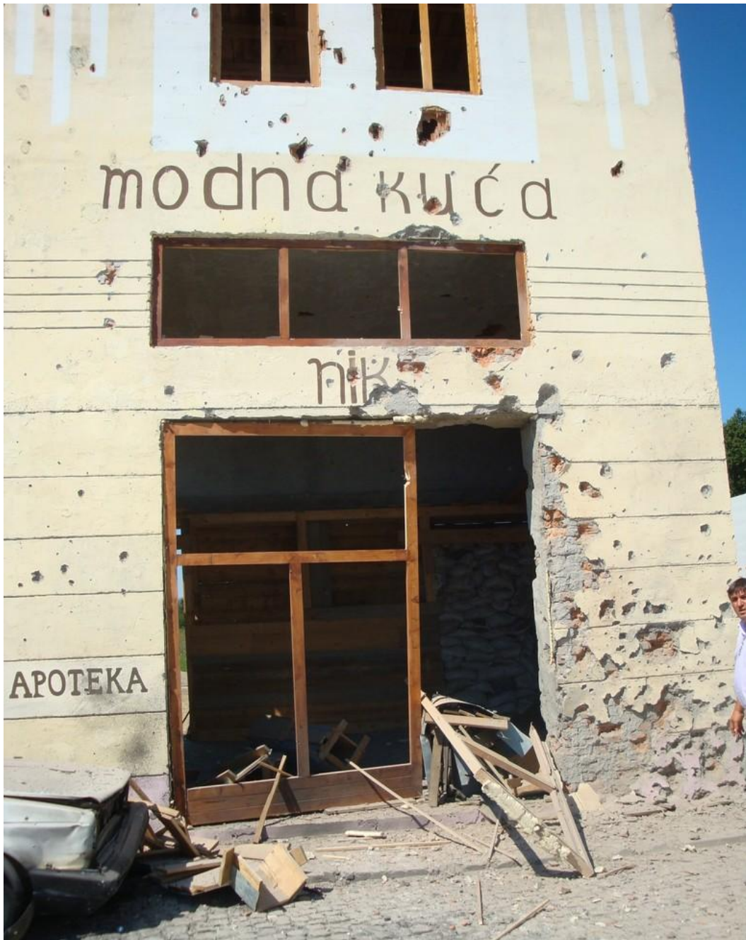
Figure 13 – Appearance of the lower right part of "NIK" store object facade, and part of facade above shopwindow
