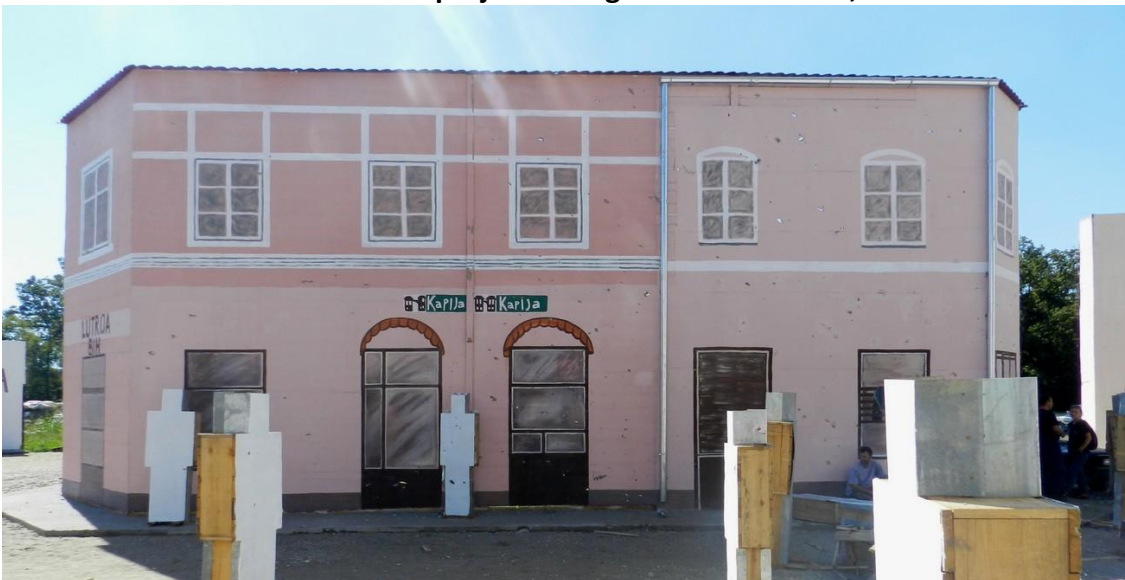
Figure 30 – Appearance of central facade part around “Kapija” premises, with visible fragmentation action traces of projectile activated during the experiment
