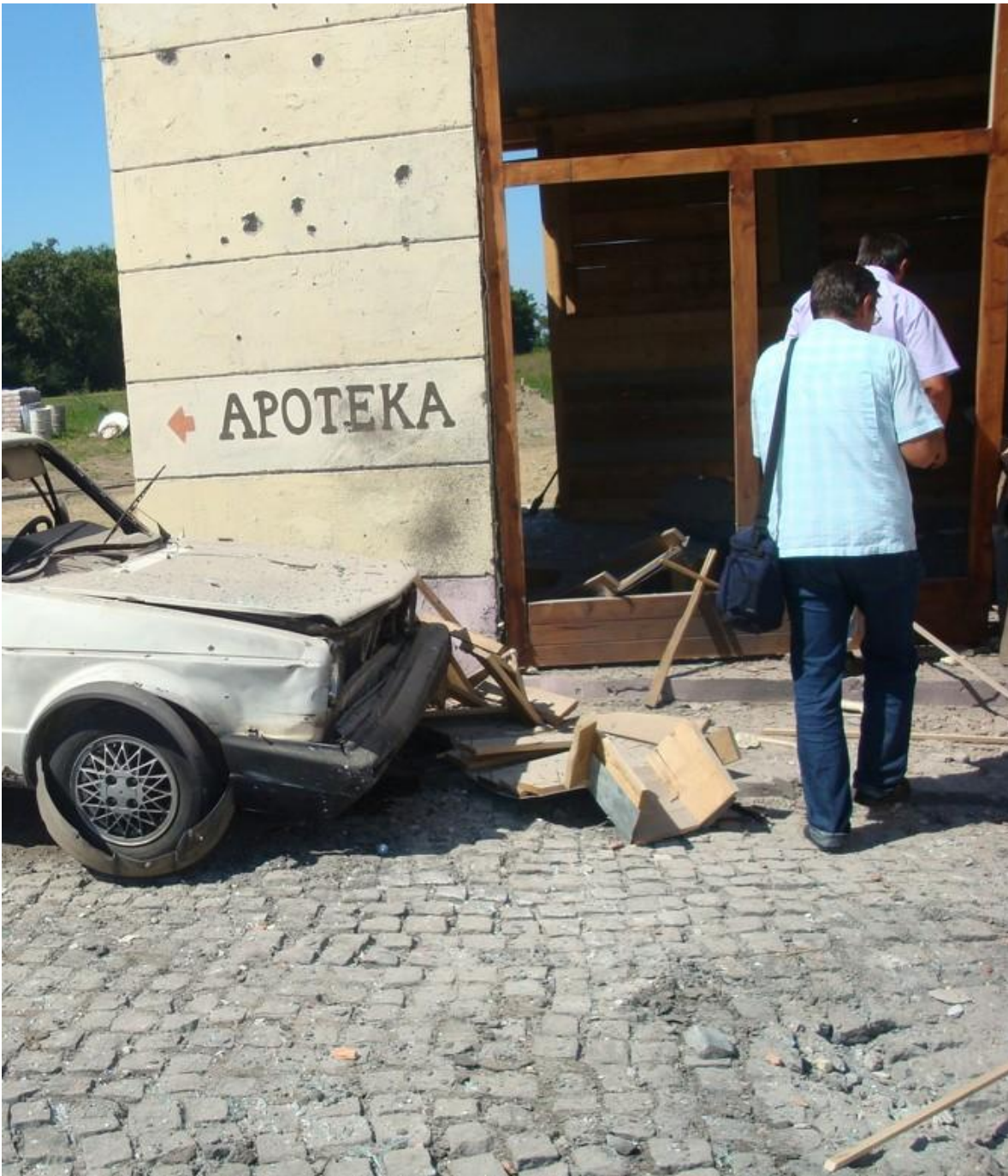
Figure 15 – Appearance of damage to the left part of "NIK" store object facade
