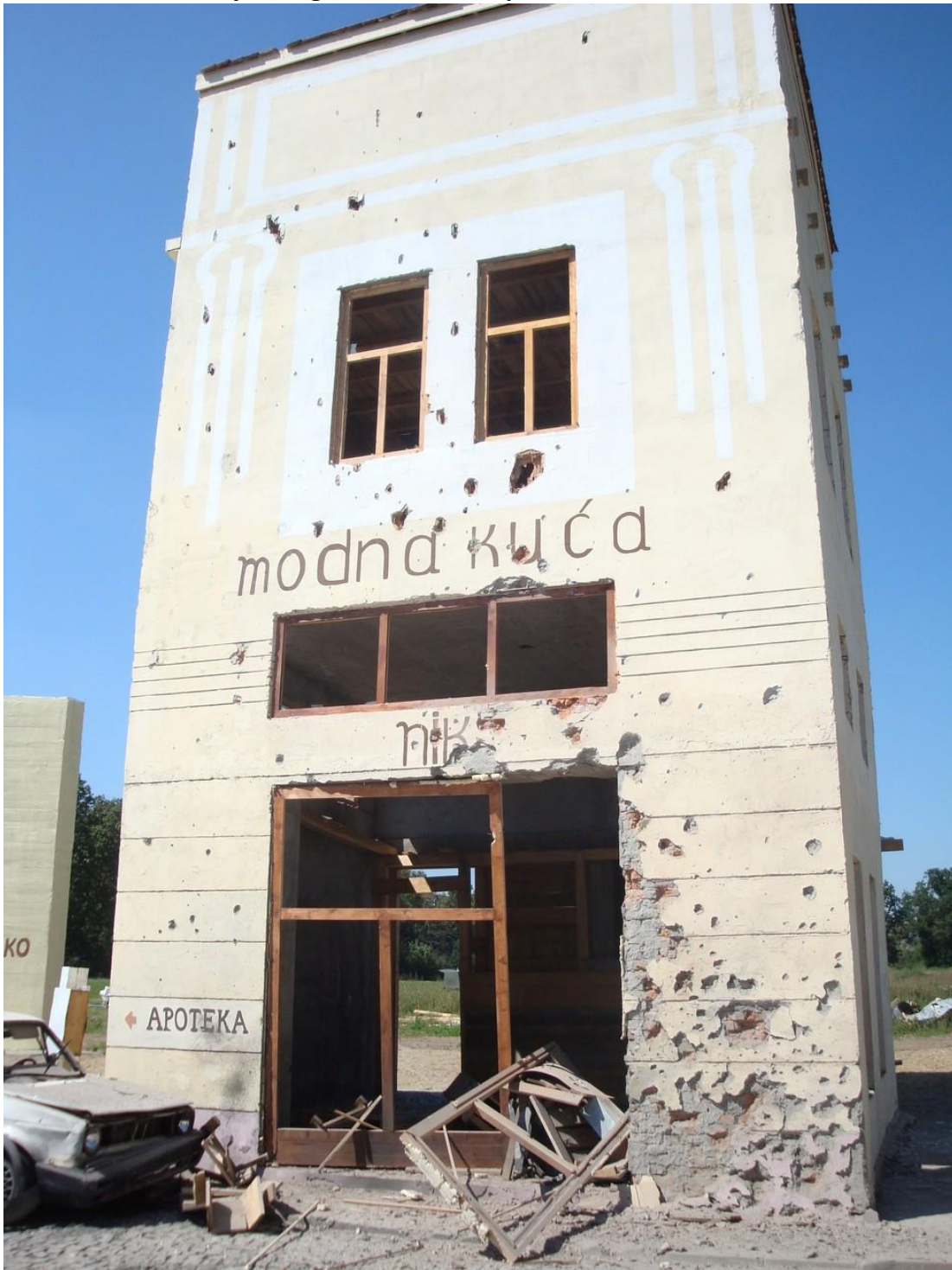
Figure 14 – Appearance of "NIK" store object facade with damage made by fragment action of the projectile
