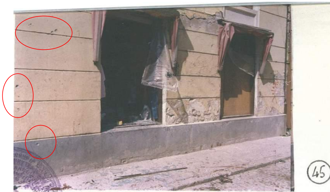
North-east side of actual NIK building after the event
