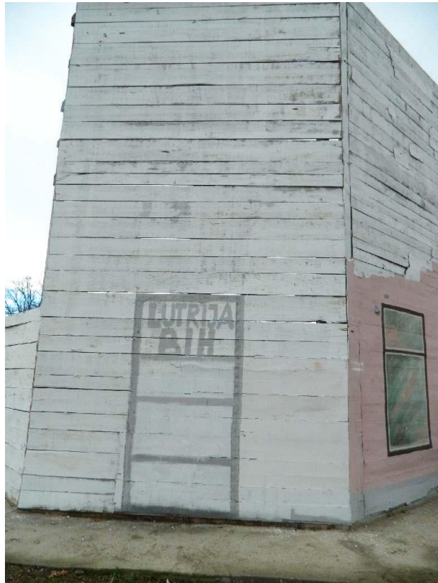
East corner of Leonardo café building (Lutrija BIH) was untouched in the experiment, which is normal since this side is not in line of sight from the explosion crater
