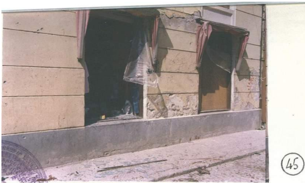
North-East side of actual NIK building after the event
