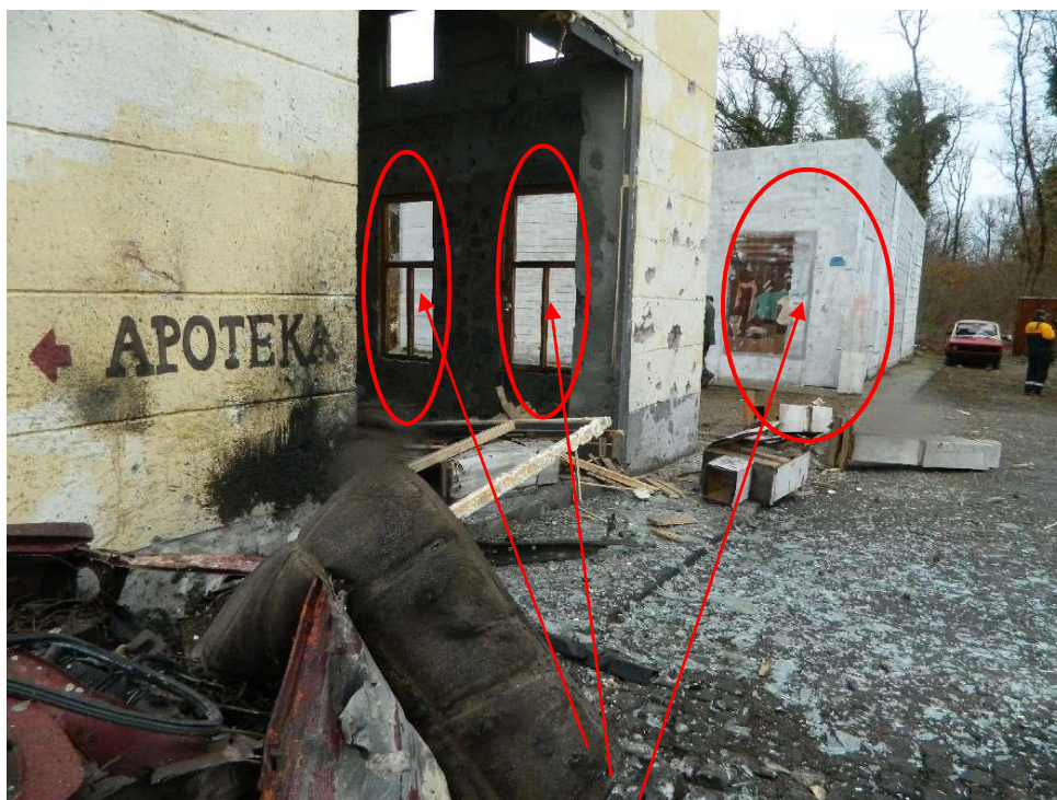
Impacts on the building across the M. Mujbegovica Street. Some fragments went through the side windows of NIK building.
