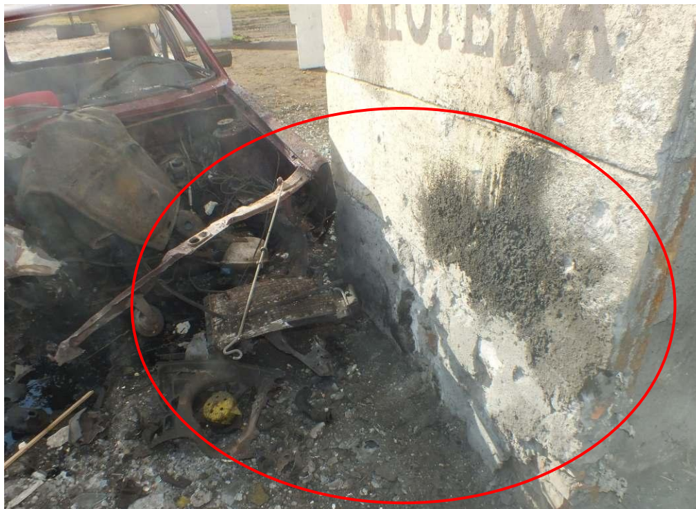
Accumulation of dirt on NIK building coming essentially for the material that was between the granite cubes
