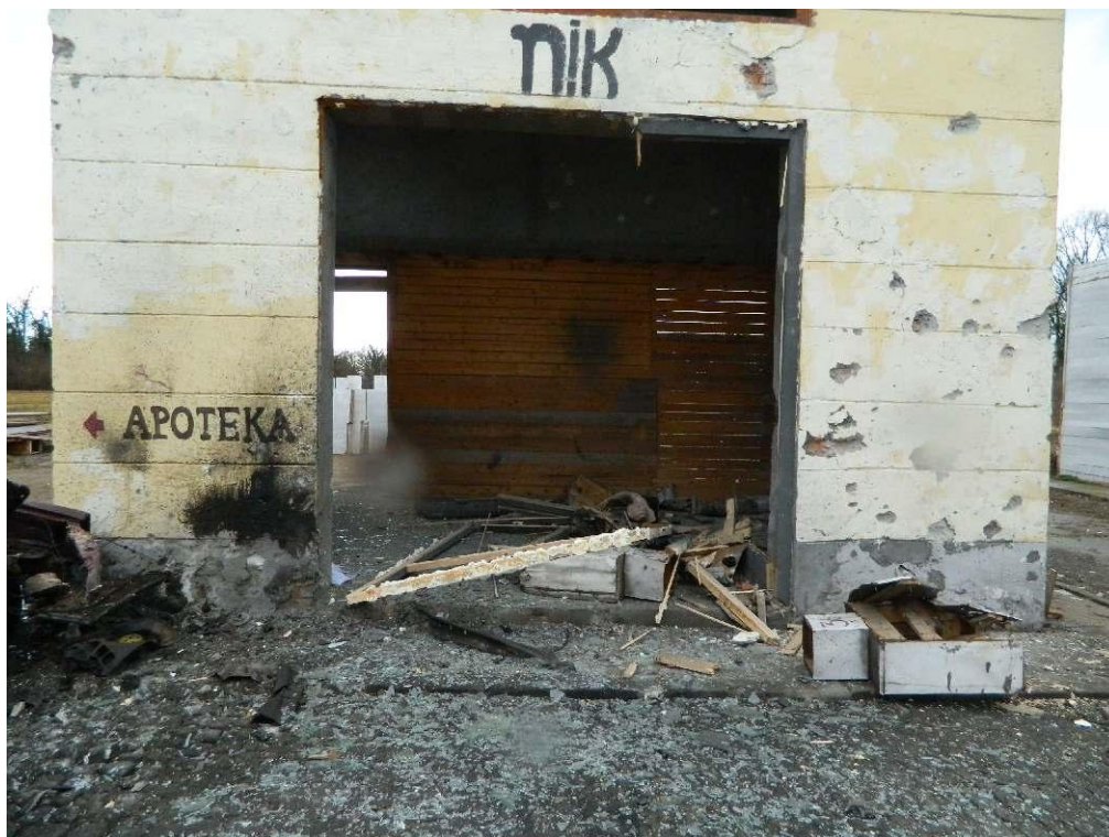
Store window of NIK building : results of explosion during experiment at NIKINCI Feb. 10th, 2016
