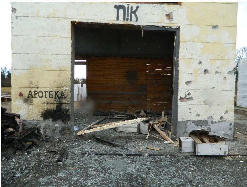
Impacts on the north side of the mock-up NIK building
